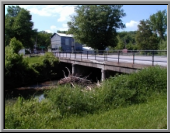
Blockage under deteriorated bridge
